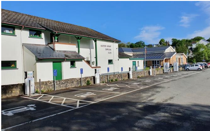
Electric charging “hub” at Saundersfoot car park
