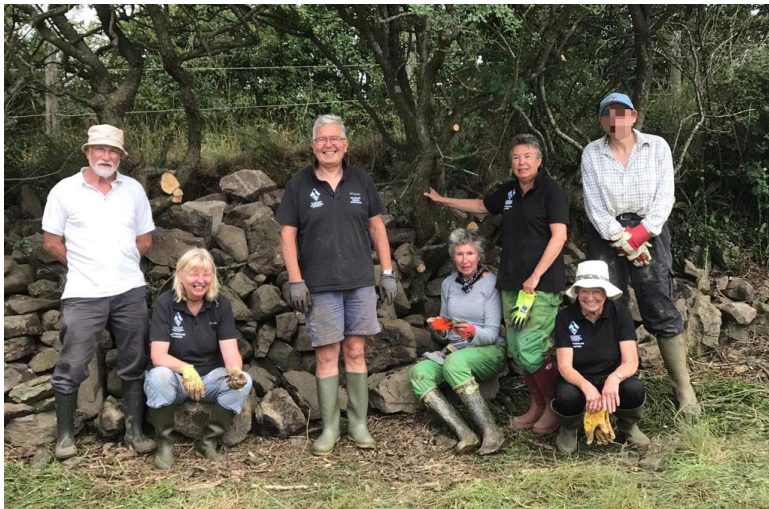
Image: Carew Volunteers building a revetment wall on the banks of the Millpond
